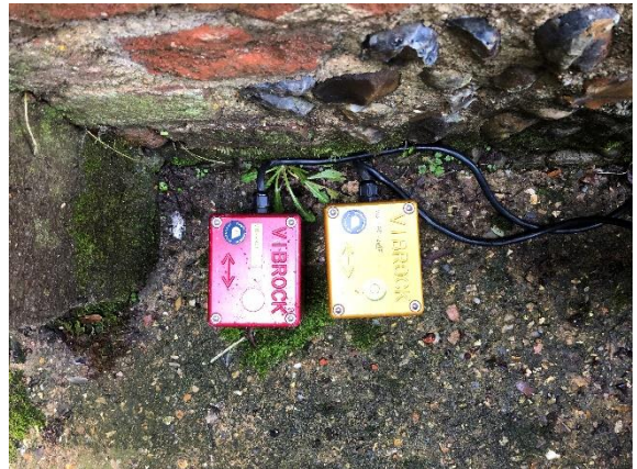
Figure 3.7: Vibration Monitor at 20 High Street
